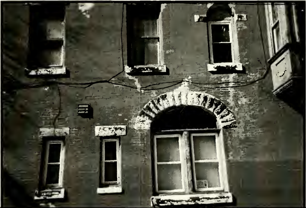
SIDE FACADE OF AN ABANDONED APARTMENT BUILDING AT MONTGOMERY AND NATRONA, STRAWBERRY MANSION, 1998.
